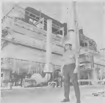
Fuels Division Superintendent Marciano "Rocky" Angela at the new crude furnace of the revamped Nos. 5 and 6 Pipelines. Rocky began his assignment with Imperial Oil Ltd. at Sarnia, Canada, February 1.
